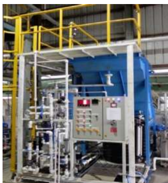
Figure 24: 10 cu.m/d Brine Purification System.
